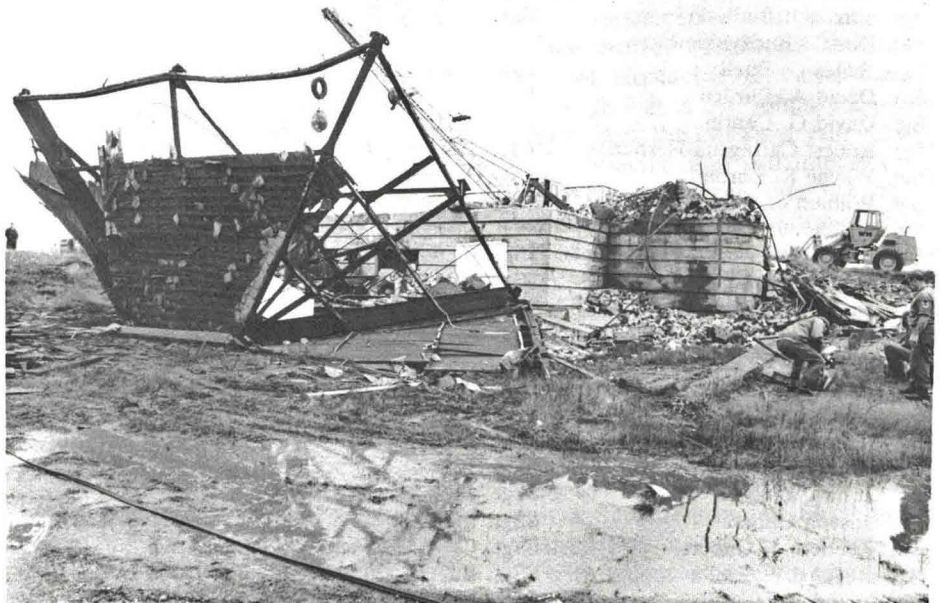
If these walls could only talk, what secrets they might divulge! Under the wrecker's ball is the former incinerator used to burn classified material when SAC units were stationed at Westover.
