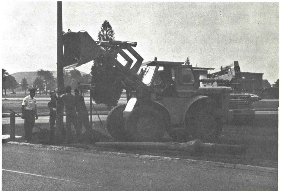
Members of the 901st CES make "light" work of the installation of new street light standards on the base ellipse on Oct 21. MSgt. Frank Notturmo supervises TSgt. Albert Drenthe, SSgt. Randy Malek and SrA. Robert Foley while SrA. James Dupuis controls the front end loader.
