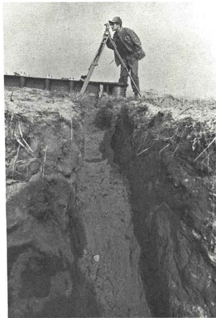
SSgt. Larry Schuller, 823rd CES, uses a transit during the construction of an arresting barrier on Westover's main runway. The anchor for the system is buried beneath the trench in the foreground.
